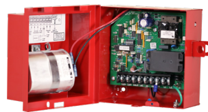
Capacitor in IQ Control Box 008800581
